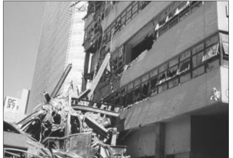
Damage to CUNY's Fiterman Hall in Lower Manhattan.
